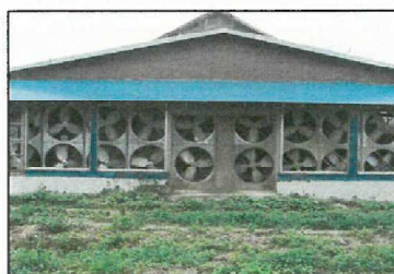
↑牛舎壁面の換気扇
