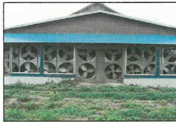
↑牛舎壁面の換気扇
