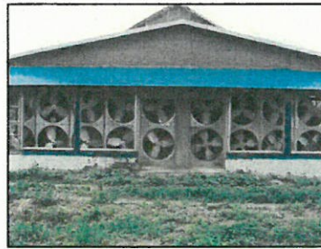
↑牛舎壁面の換気扇
